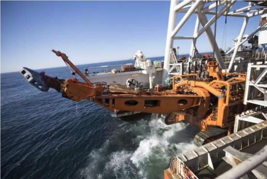
The giant subsea "crawler" tractor is lowered into the ocean from the deck of the Mafuta.
